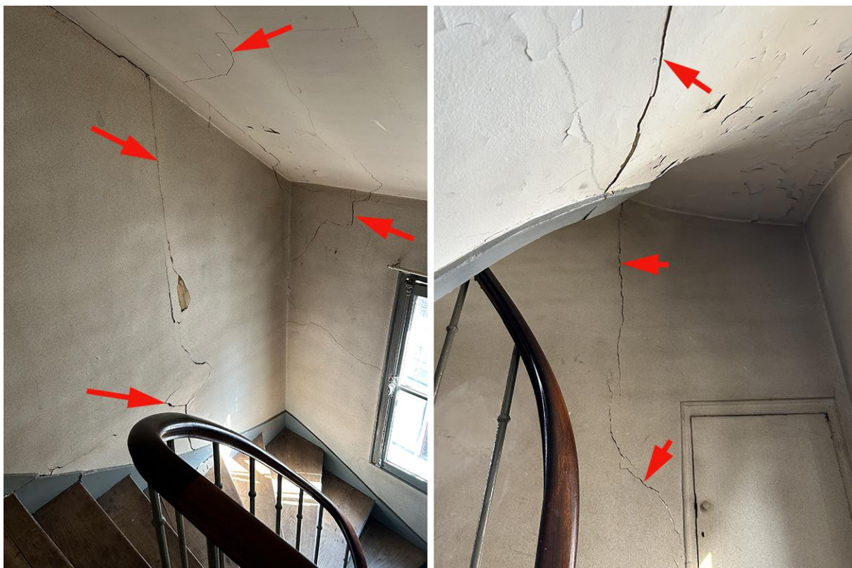
Fissure R+1 / R+2
